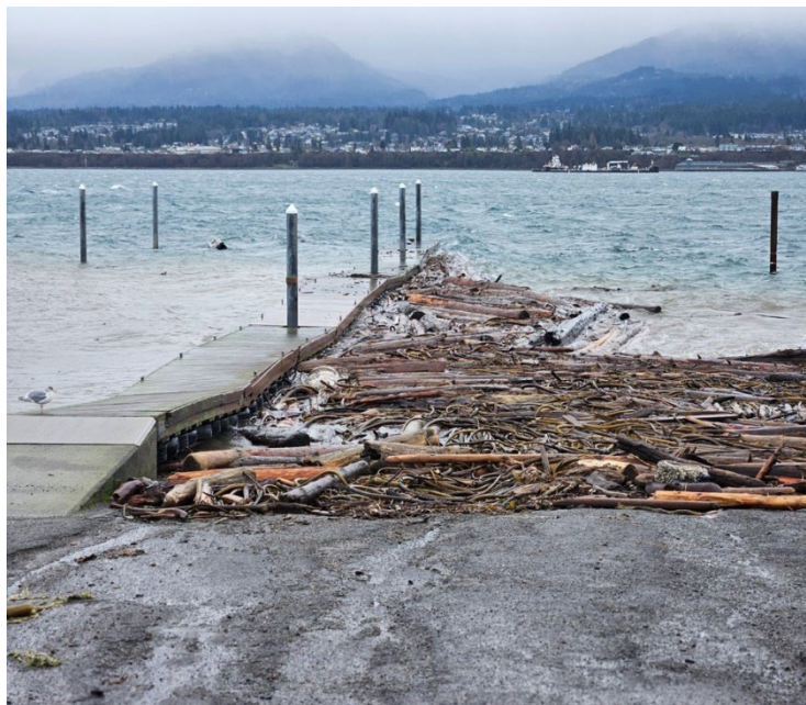
Figure 2 Boat launch damage caused by storm-driven waves.
