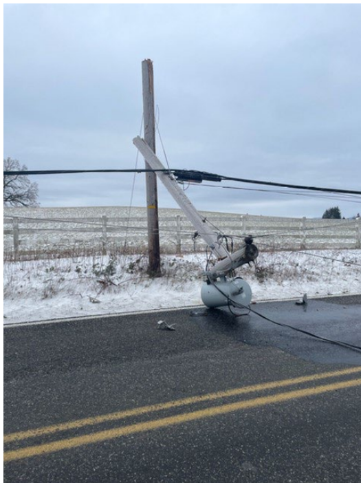
Figure 3 A utility pole knocked down and lines across a public road in Cowlitz County.
