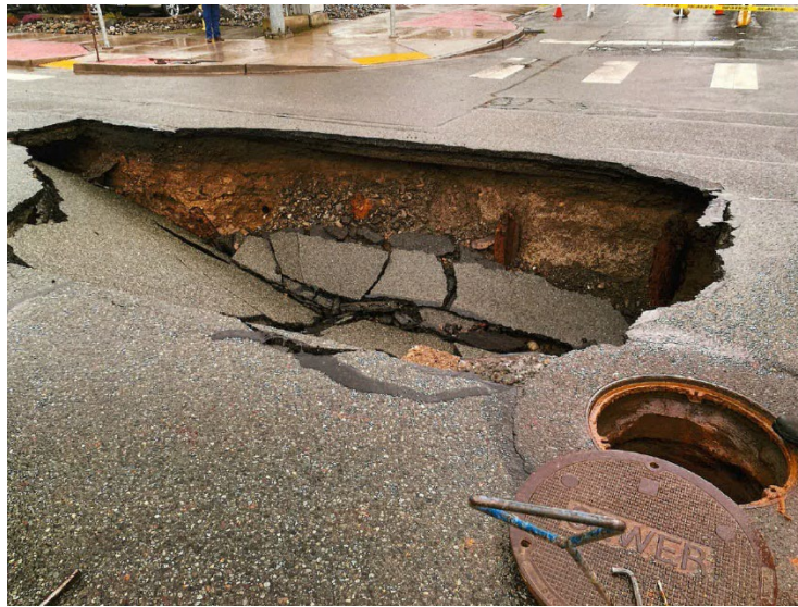
Figure 1 A sinkhole caused by excessive rains and subfreezing temperatures on a main public street in Clallam County.
