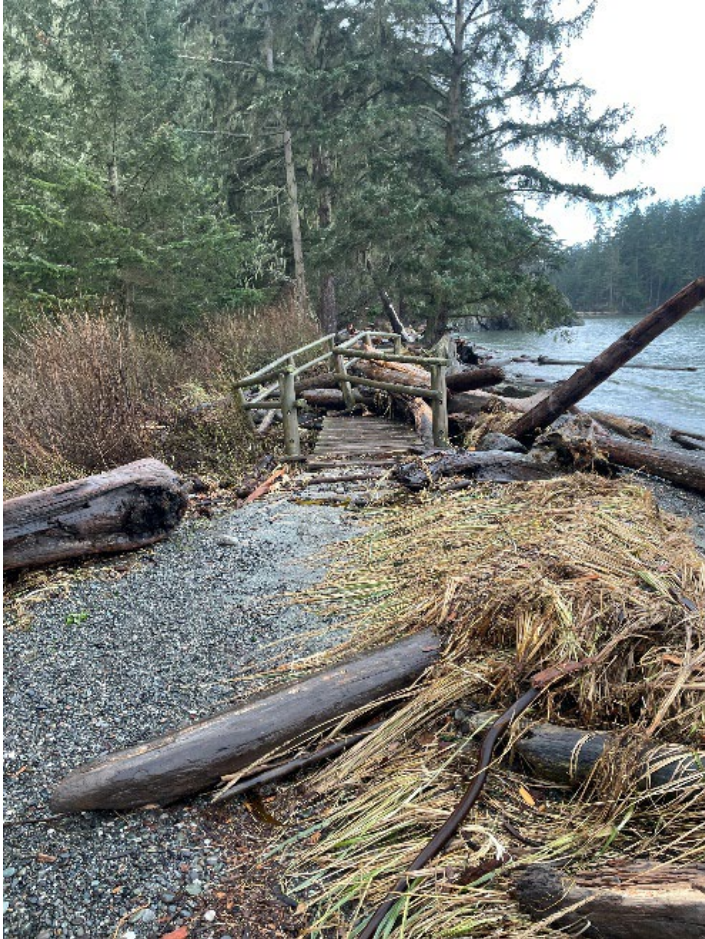
Figure 13 Damage to a wooden pedestrian bridge at Deception Pass State Park.
