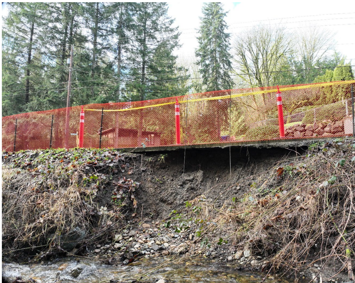
Figure 9 In the city of Kenmore, a roadway sustained severe erosional undercutting by excessive rains and stormwater runoff.
