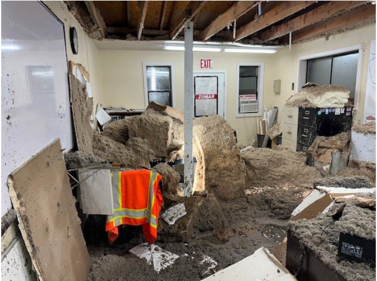
Figure 10 The Lewis County public works building was flooded and severely damaged by burst and frozen pipes.
