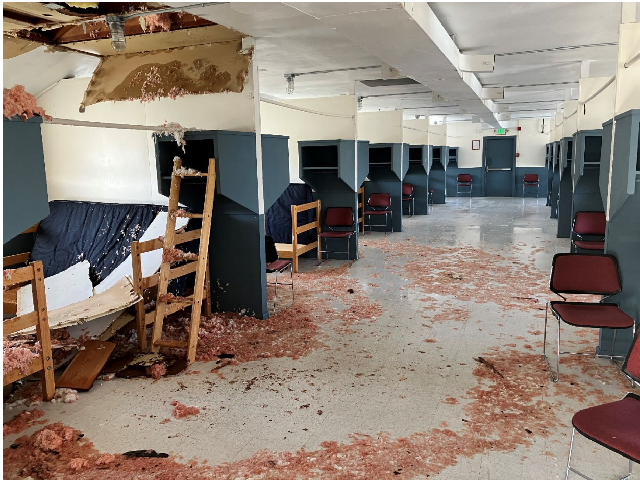
Figure 6 Burst pipe damages at Fort Flagler
